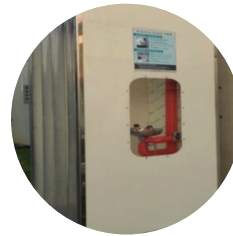
Outdoor emergency washing facility
