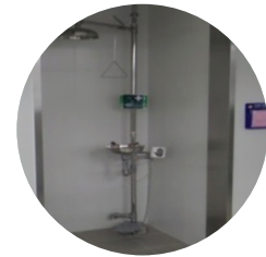
Indoor emergency washing facility
